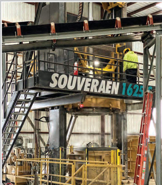
Installation crew finishing the setup of the BFS Souveraen 1625 S at The Turner Co. plant in Lockhart, Texas.
