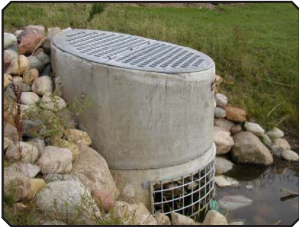
Pond Skimmer with Manhole Side Grate
